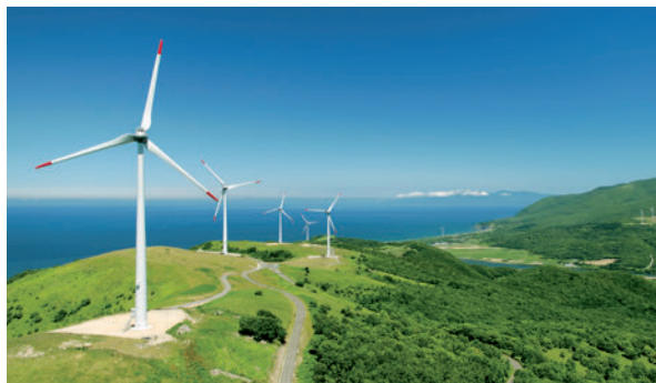
Shiribetsu Wind Power Plant (Hokkaido)
